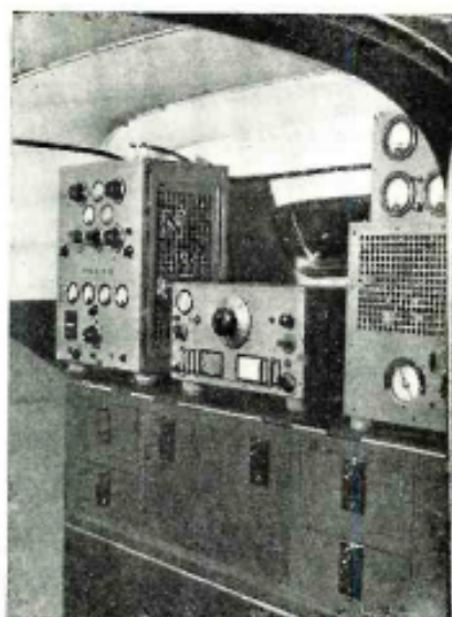
Everything tied down and within reach to insure efficient operation.
